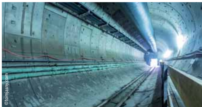
Utility fixings in TBM tunnels with curved anchor channels
