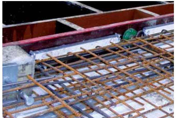
Installing HALFEN HTU Cast-in channels in the front face of a slab
