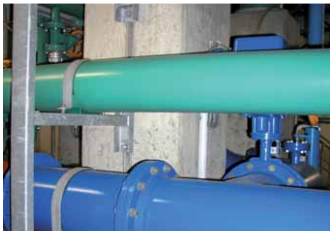
Pipe supports on vertical HZA Channels
