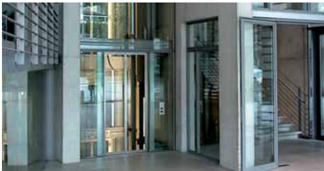
Lift fixings, guide-rails
